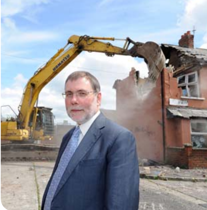
Minister for Social Development Nelson McCausland MLA at the demolition of houses at The Village, Belfast.
